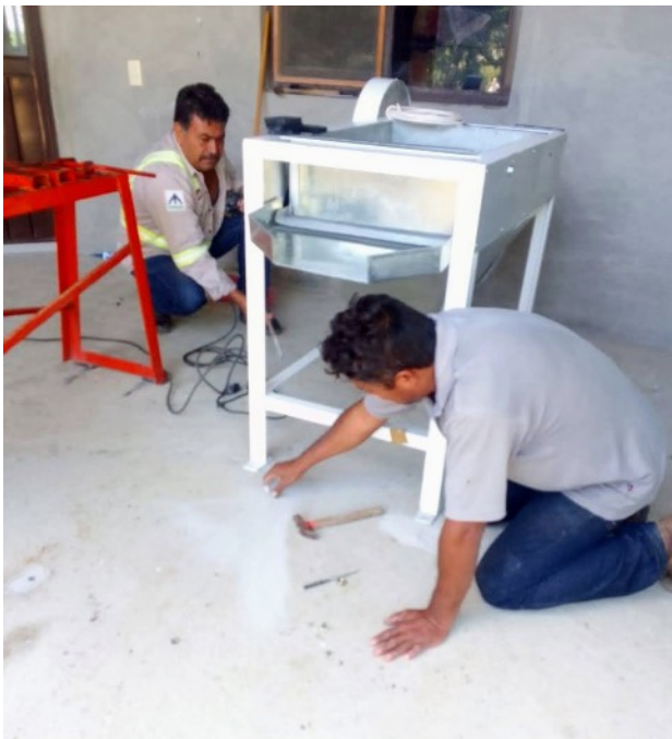
Above: Drying the new materials delivery pathway; Right: Installing the new sieving machine.
